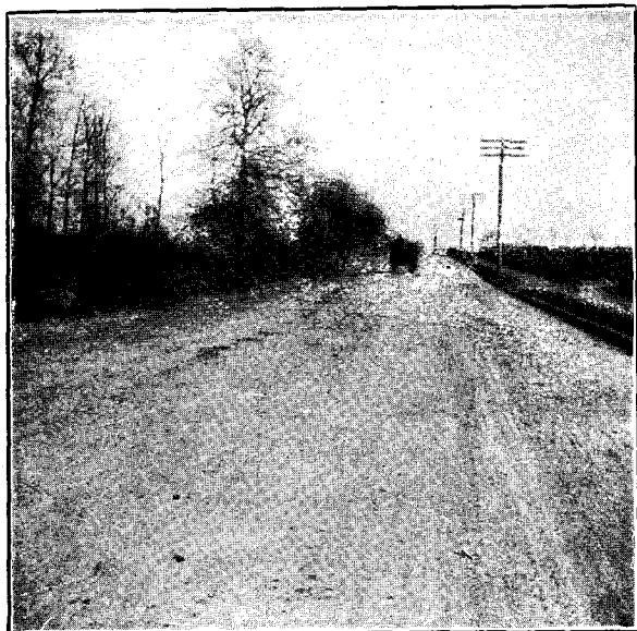
(b) Same road after completed and rolled with steam roller. See page 950.
