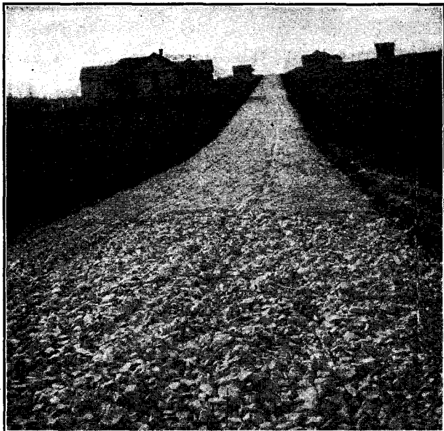
View on Eleventh Street and Vernal Pike extension, showing foundation stone and placing of top dressing.
