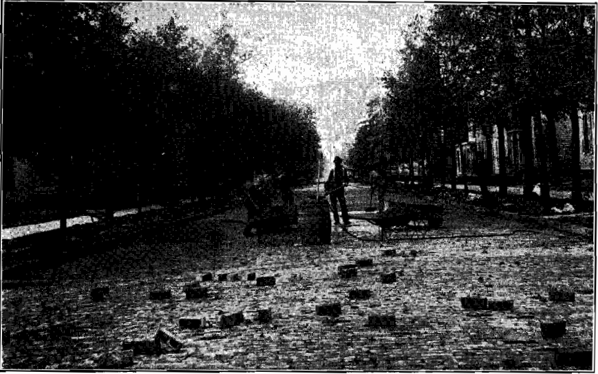
The last Inspection of the Brick before the Application of the Filler.
