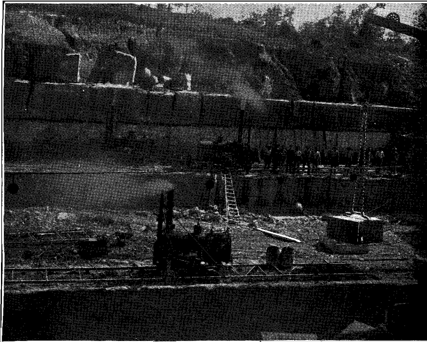
2. In new quarry, looking south of east, showing method of quarrying, thickness of covering and regularity of the upper surface.
